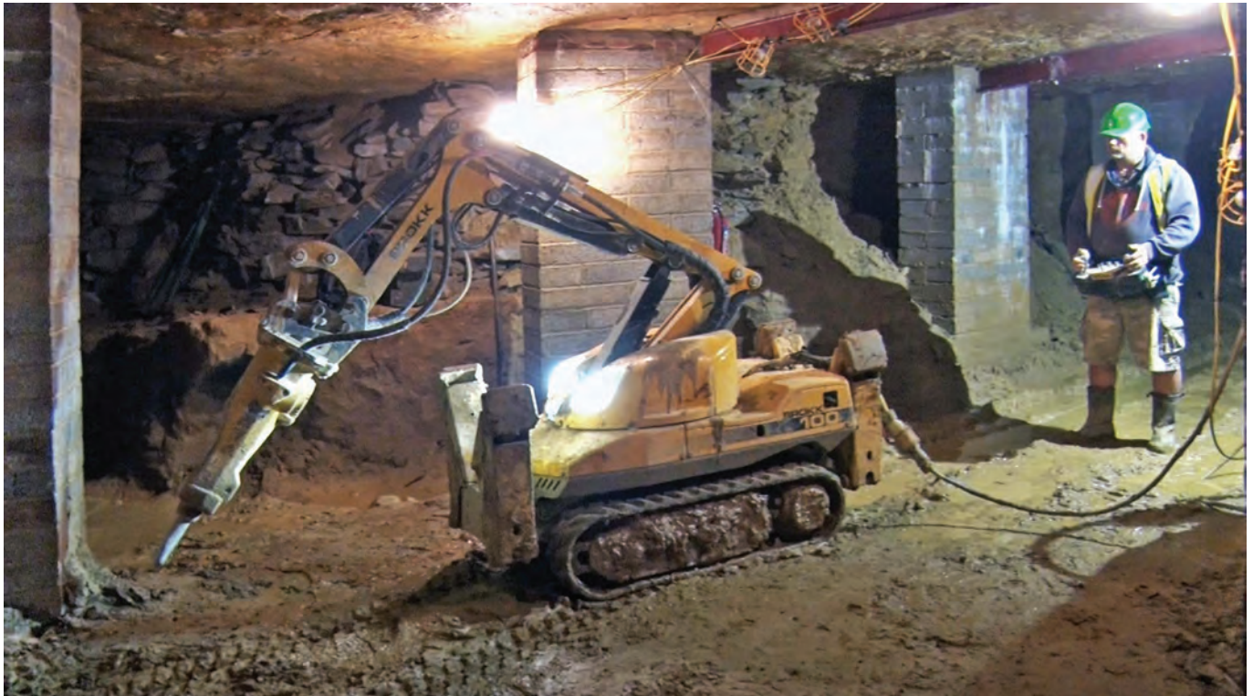
Brock-100 mounted remote-control jack hammer operating in Claude Smith's reopened mine at Collyweston
